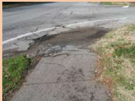
Large pothole creates hazard on Pendleton Road bike path
