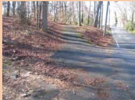
Tree roots create uneven surfaces on Edgewood Avenue, Pendleton Road, and Old Central Road
