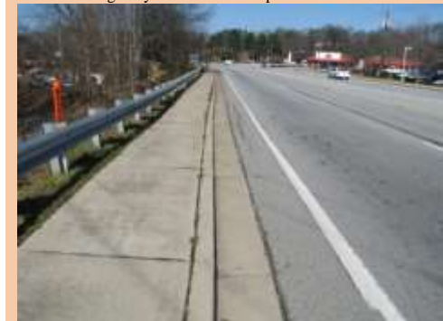
Highway 76: Fails to meet AASHTO standards regarding dedicated bike lanes.
